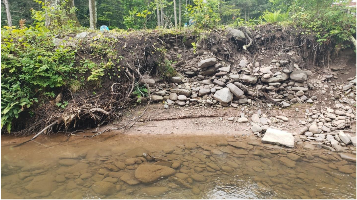
FIGURE 3. EROSION INTO ALLUVIAL BANK WITH LACUSTRINE EXPOSED IN TOE.
